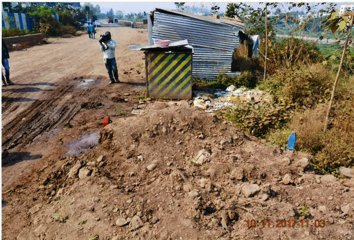
This entire road needs to be demolished and shifted away from the river bed (chainage 400M to 750M)
