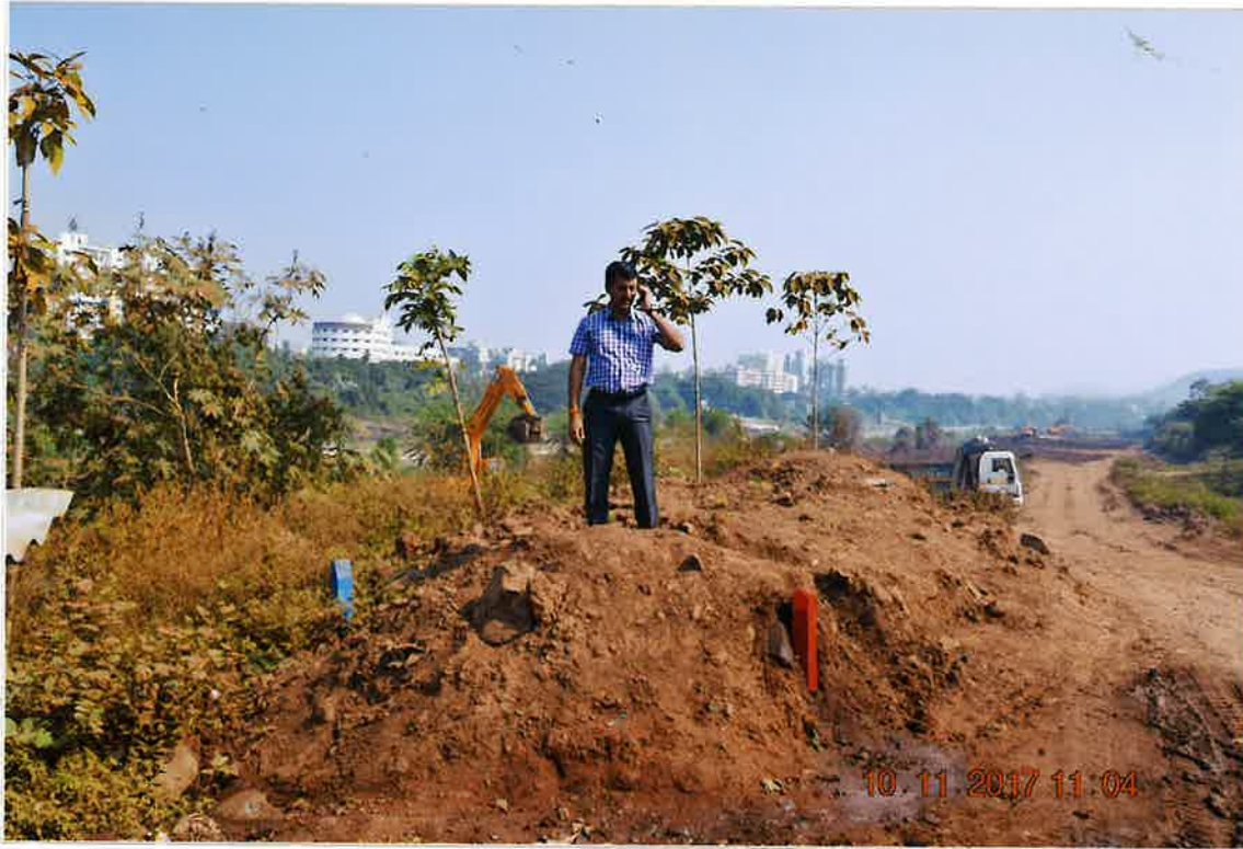
Erroneous flood line marking at site at chainage 750M. Note - Red Flood line and Blue Flood line shown at the same level.
